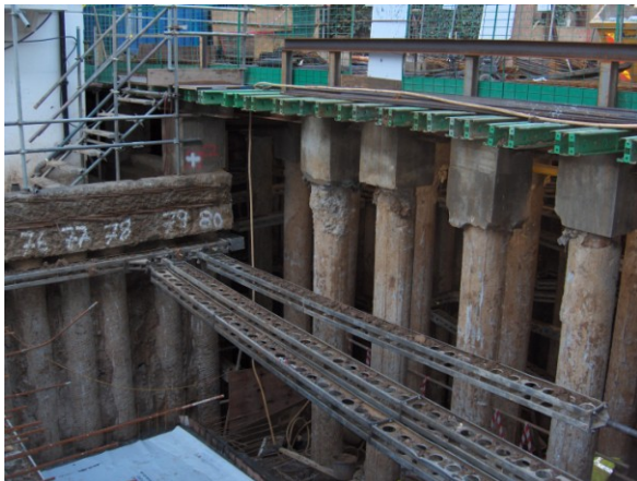
The temporary steel shown in this image on top of the load bearing piles is to enable the excavator access to dig out the basement.
