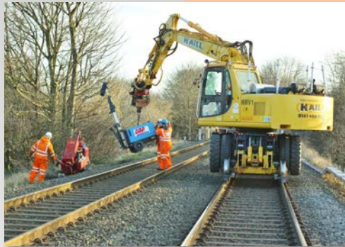
Plant and materials were moved to the work areas using road rail vehicles (RRVs) and trolleys
