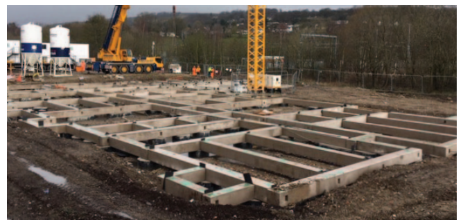
Van Elle's largest Smartfoot installation working at a rate of 200 linear meters per day
