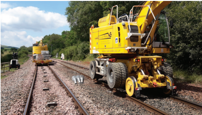
Kirkconnel track bed stabilisation project Glasgow and South Western Railway (GSW) Line.
