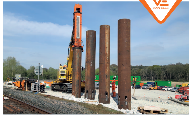
Highlands Enhancement Project (Don Viaduct) - Installation of CFA piles and CHS piles for Bam Nuttall
