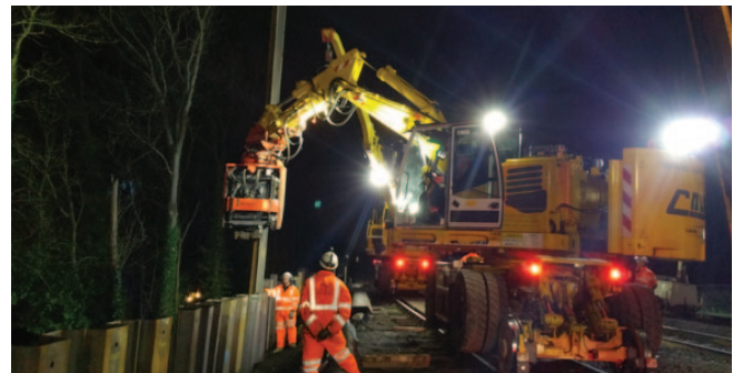
Maidenhead retaining wall Crossrail Western Outer Track Infrastructure on behalf of Balfour Beatty
