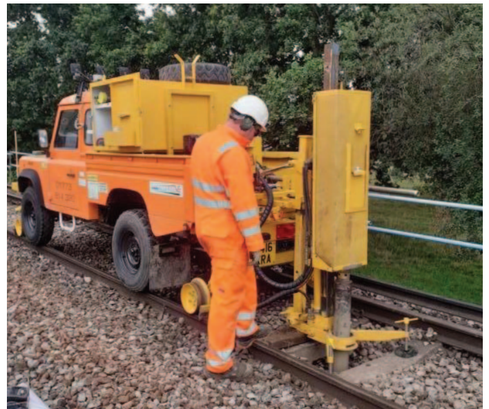
Van Elle's RRV Land Rover pictured, here in Wokingham, incorporating the dynamic sampling mast to its load bed. Capable of carrying out self sufficient ground investigation within the four foot of the track.
