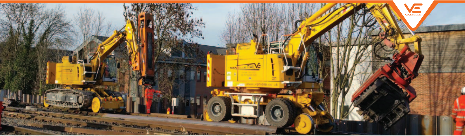
Maidenhead retaining wall for Balfour Beatty Rail utilising sheet piles, OLE, anchors and on-track civils
